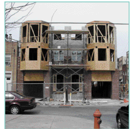
Sixteen single-family homes, marketed for between $299,000 and $410,000, are under construction on the site of the former Palumbo's restaurant at 9th and Catherine Streets in Bella Vista.
